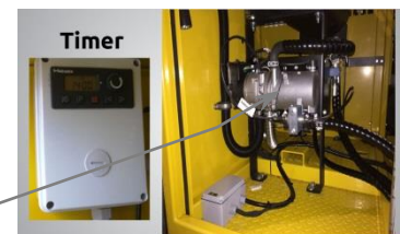
HEATING SYSTEM FOR LUBE OIL TANK
